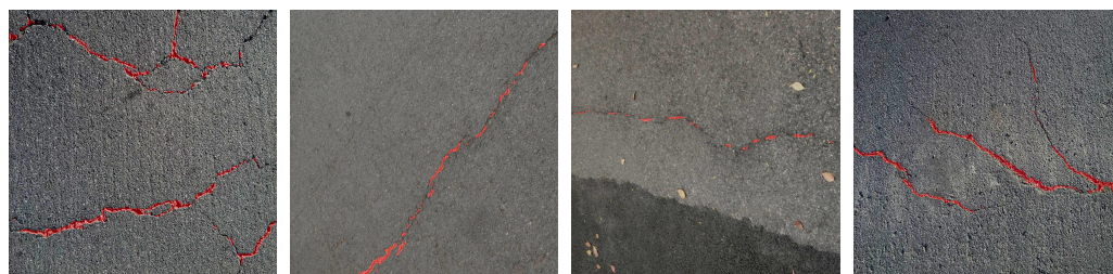
Figure 1. Segmentation results of pavement cracks, the red mask portion represents the segmented crack area.
