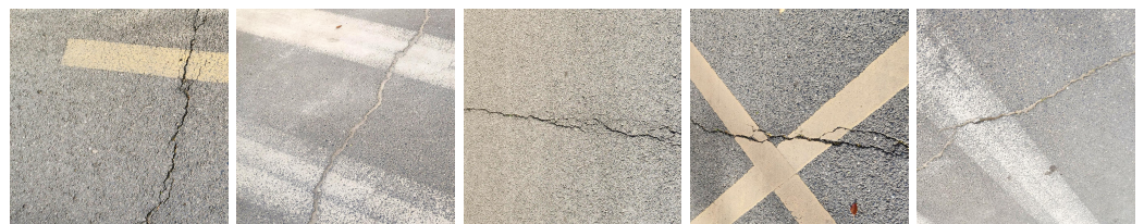
Figure 7. Pavement crack image data collected on campus.
