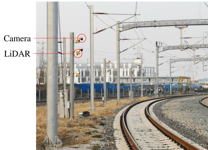
Figure 8. Railway monitoring equipment.
