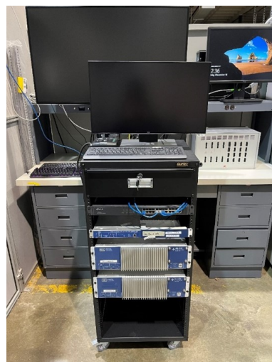
Figure 6. Strata Grid system in RPI Lab.
