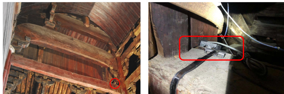
Figure 1. Installation point of tenon displacement sensor. The sensor mounting position is marked in the picture with a red circle and a red box to make it clearly visible.
