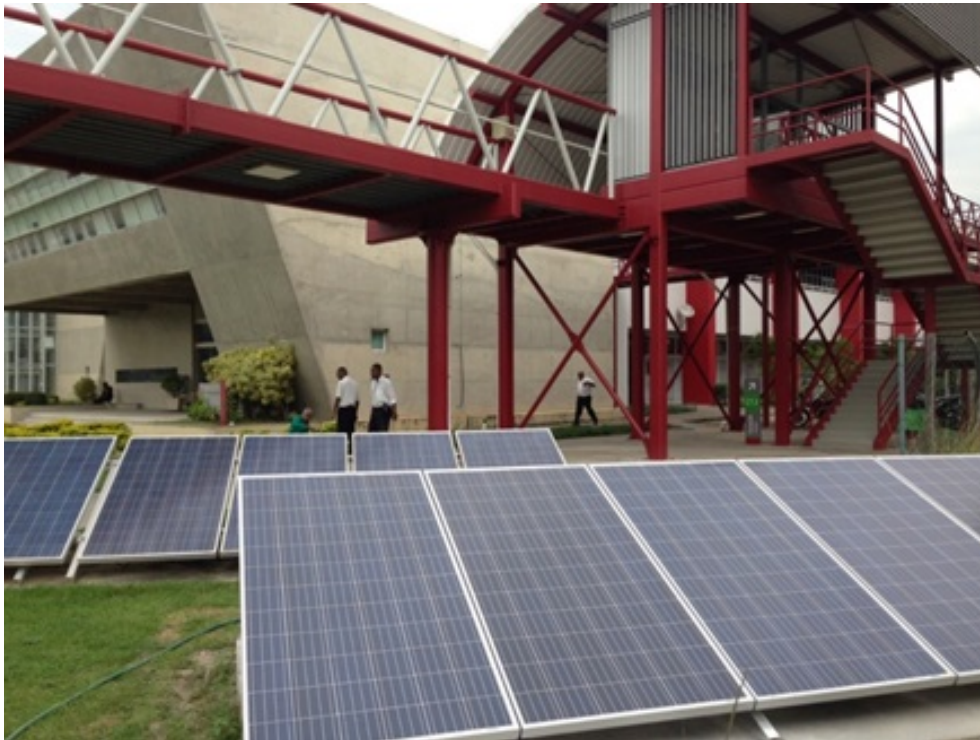
Figure 8. Twelve solar panels of 250 Wp each (total of 12 kWh/day).
