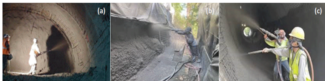
Figure 1. In (a,c), the construction of tunnels is depicted, while (b) shows the construction of ground support walls. All images feature exposed reinforcement bars and highlight the labor-intensive process of spraying concrete (shotcreting) to fill the surface [9].
