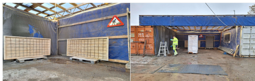
Figure 7. The semi-indoor scene in Denmark serves as Testbed 02, situated within the construction site. Here, wooden frames with exposed reinforcement bars are prepared for shotcreting.
