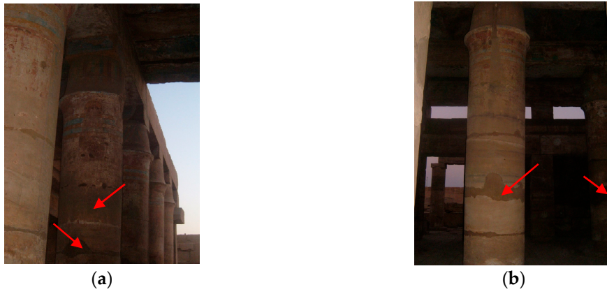
Figure 7. Deterioration in the walls of El Karnak temple (a,b).
