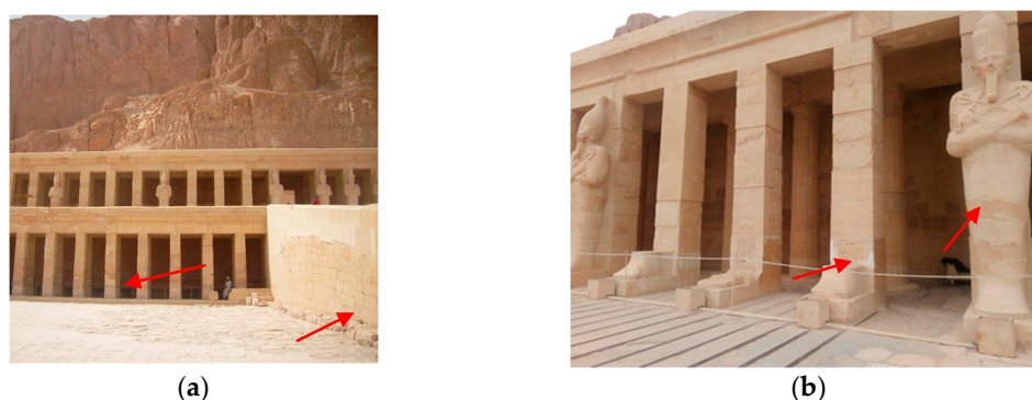
Figure 10. Deterioration in the inscriptions and writings in the walls of Hatshepsut temple (a,b).
