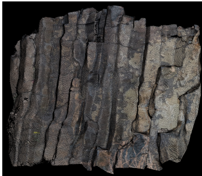
Figure 30. 3D visualization for the fusion of spatial information of TLS point cloud and texture information of digital images.
