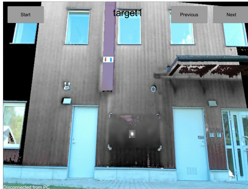
Figure 4. A screenshot of the application running on the tablet viewed by users. Notice the façade region is replaced by IR information due to chroma keying composition and the IR image of target No. 1 (the bright spot between the two doors) is correctly registered with the visible video frames.
