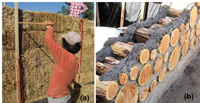
Figure 5. (a) Straw bale load-bearing wall, and (b) cordwood wall construction (credit to Wikimedia Commons).
