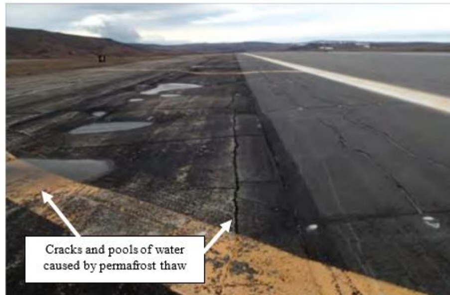
Figure 1. Cracked runways at Thule AFB, Greenland, from permafrost thaw and refreezing adapted from [39].
