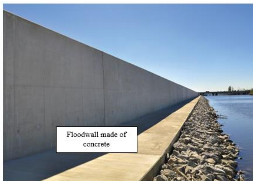
Figure 9. Floodwall along the coastline adapted from [80].
