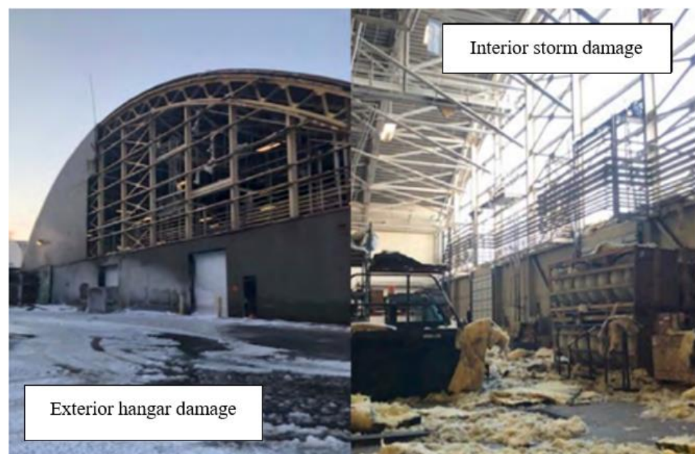
Figure 2. Storm damage to hangars at Eareckson Air Station, Alaska adapted from [39].
