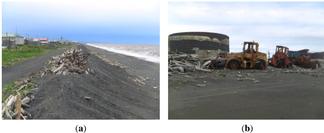
Figure 4. (a) Berm construction efforts in Shaktoolik include piling up driftwood, and (b) other material including scrap front-end loaders, in an effort to construct the protective berm. Work continues to cover and backfill the berm with gravel. Photo credit: Jon Rosales.
