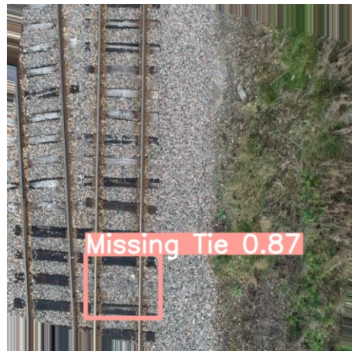
Figure 18. Positive missing tie detection.
