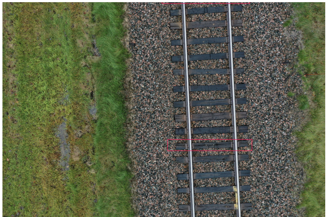
Figure 8. Example of a broken tie.
