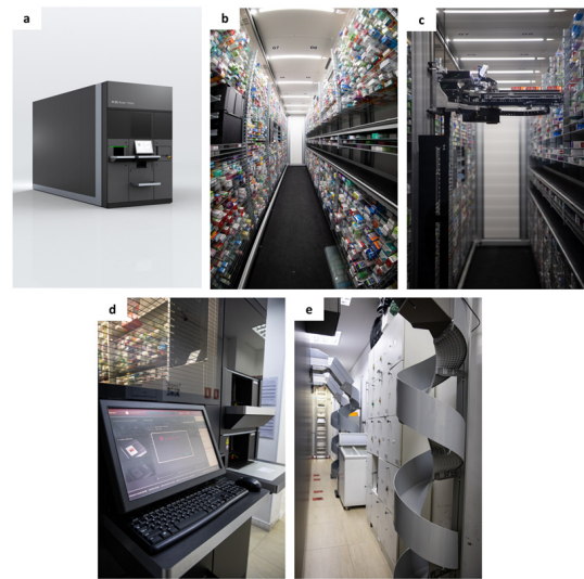
Figure 1. Robotic dispensing solution implemented. (a) Outside view of the automated storage and dispensing robot; (b) packages organized on shelves inside the robot; (c) picking head moving multiple packages; (d) touch-screen user interface and input belts; and (e) conveyor system with spiral chutes to transport packages from the upper floor to the ground floor.
