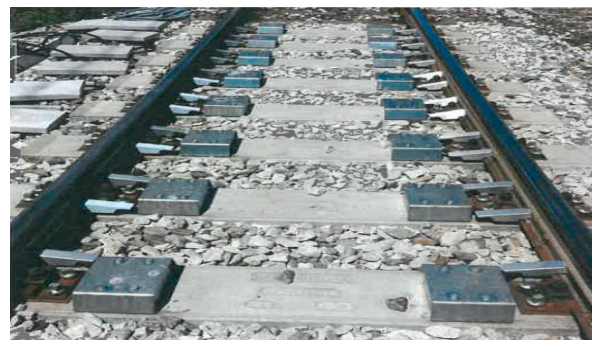
Figure 6. Layout of the Marini SMCV measuring system on the railway track.
