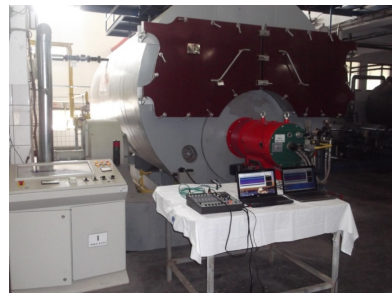
Figure 1. Boiler under measurement and test set-up.
