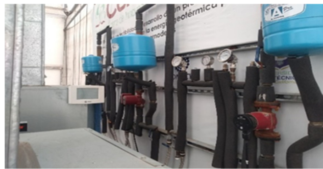
Figure 1. Geothermal heat pump hydraulic system installation in the greenhouse.
