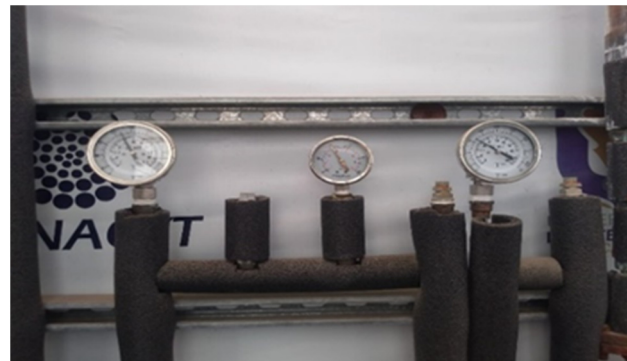
Figure 2. Analog instrumentation in the geothermal heat pump analysis was installed.
