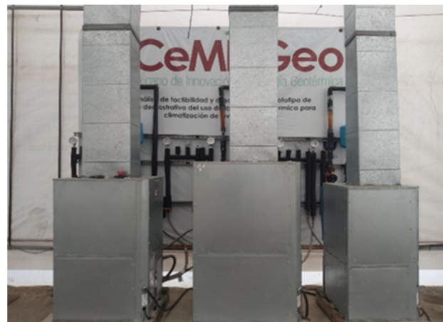
Figure 7. Geothermal heat pump systems were installed at the study site.
