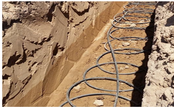
Figure 3. Slinky-type geothermal heat exchanger installation used in the GHP to assist the greenhouse.
