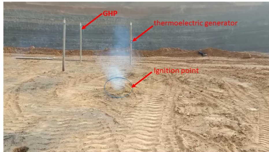
Figure 12. On-site remediation of the Maoergou coal gangue hill and temperature difference power generation.
