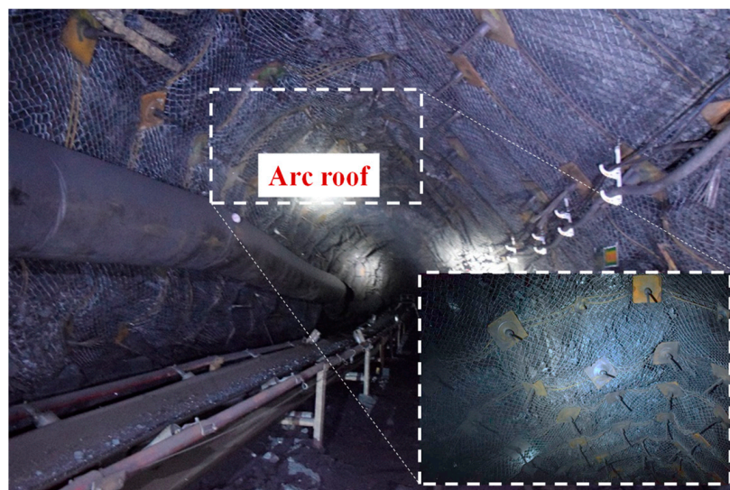
Figure 18. Maintenance and control effects of the roadway under the new support.
