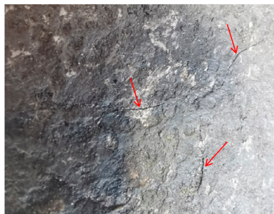
Figure 2. Macroscopic appearance of cracks and corrosion pits on the external surface (The arrows point to the cracks).
