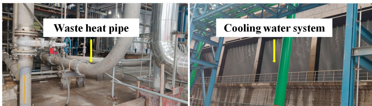
Figure 1. Image of a high-temperature industrial pipe and cooling water system in a chemical plant.
