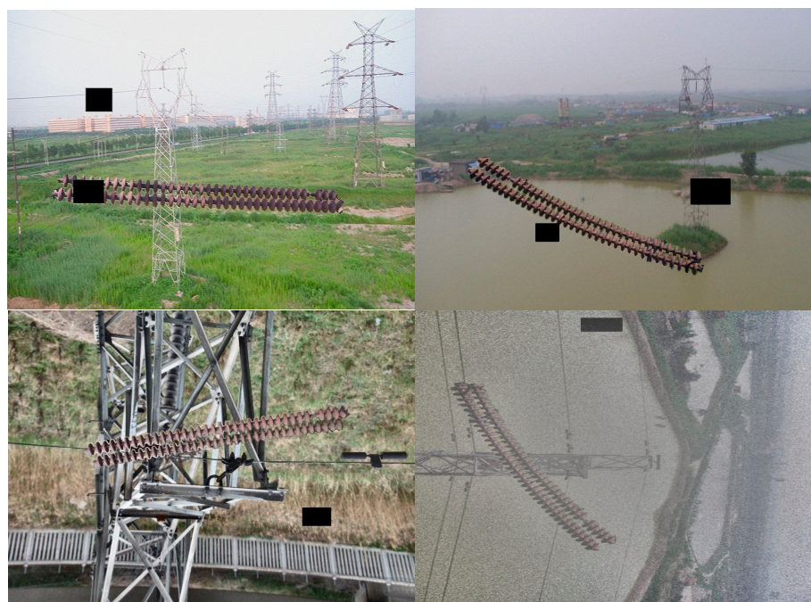
Figure 8. Part of the insulator self-explosion defect data.
