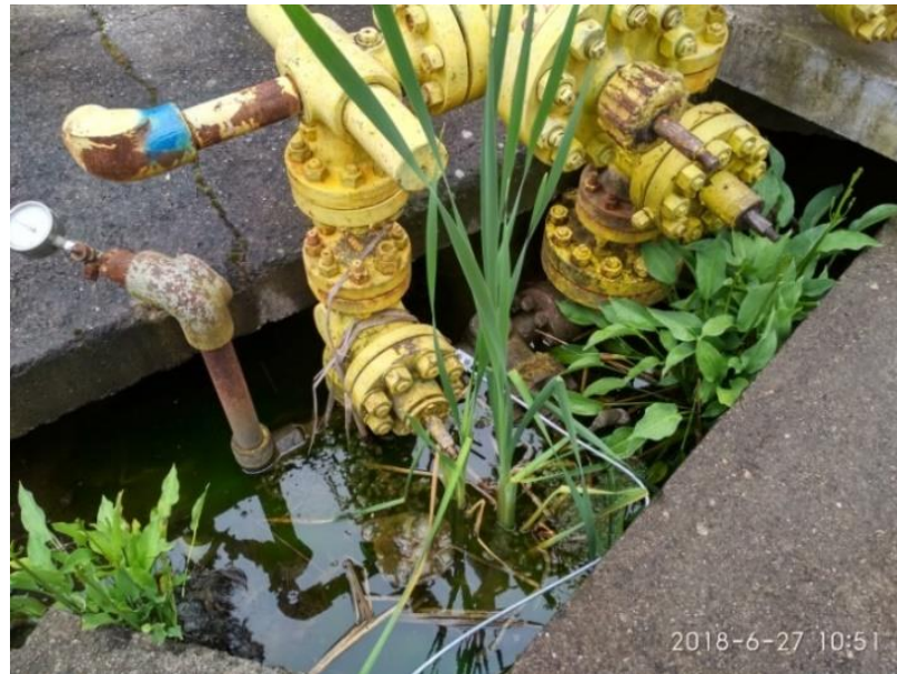
Figure 9. Example of the unsatisfactory condition of a gas well at its mouth, (source: elaborated by authors).
