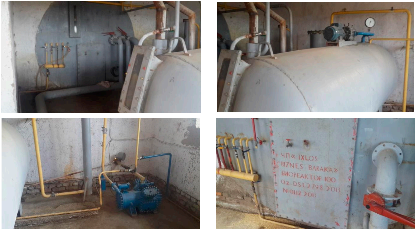
Figure 2. Biogas plant of the Agrofirma.
