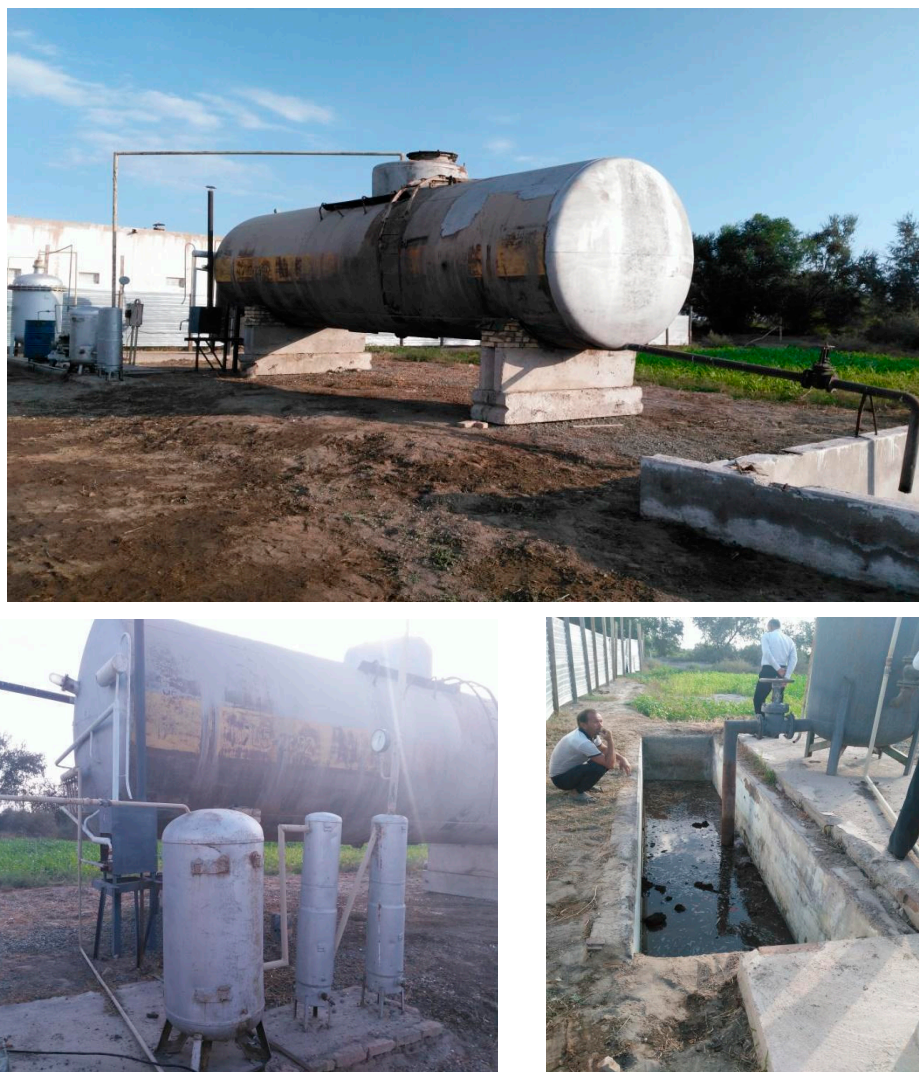
Figure 4. Biogas plant at Biougit Limited Liability Company (LLC).
