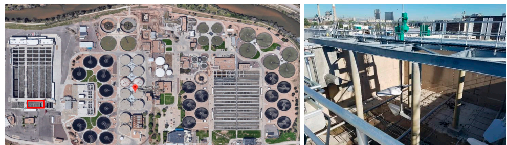
Figure 5. Photo of the ANITA Mox reactor in Denver retrofitted into an existing RAS reaeration tank.
