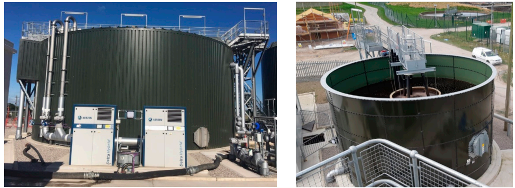
Figure 10. New IFAS ANITA Mox reactor at Wrexham ( left: IFAS tank, right: clarifier).
