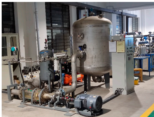
Figure 5. Spiral axial-flow multiphase pump test bench system.
