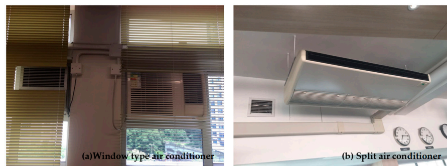
Figure 2. (a) Window-type air conditioner and (b) split air conditioner.
