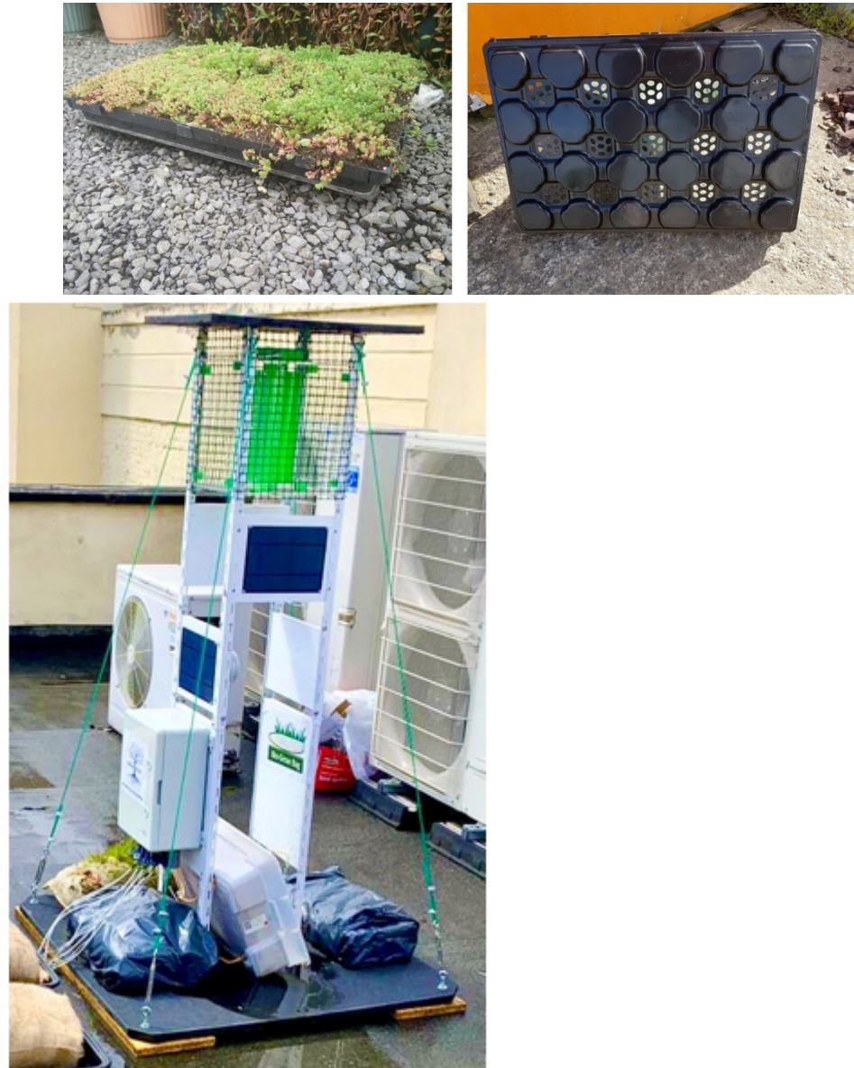
Figure 3. Green roofs and sensors in the CHQ building.
