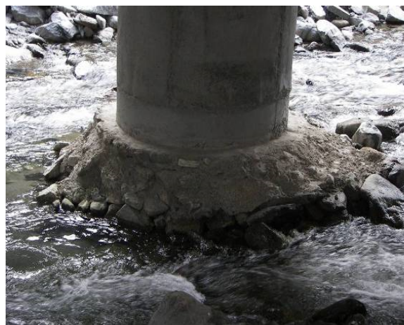
Figure 2. Local scour near longitudinal bridge piers.
