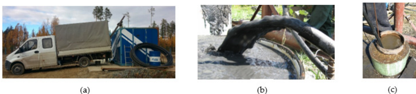
Figure 14. Well rehabilitation operations: (a) cleaning setup, (b) mixture pumped out of the well during the cleaning, (c) submerged nozzle holder on high-pressure hose.
