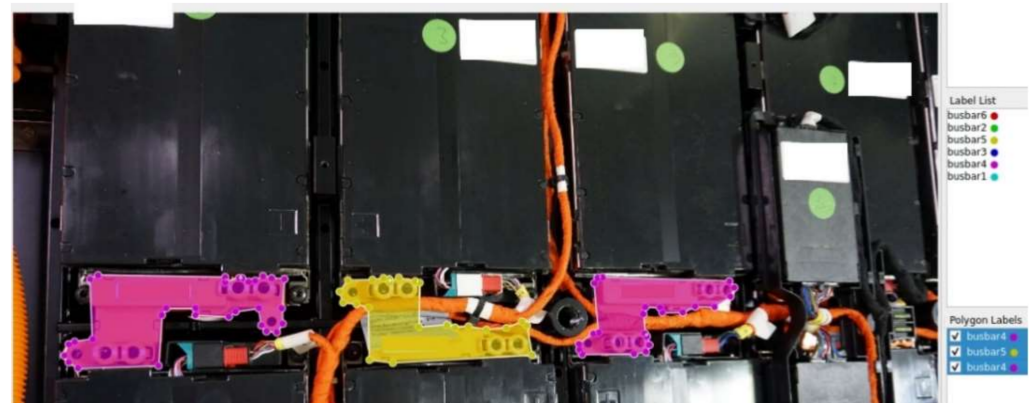
Figure 9. Annotation for instance segmentation with Labelme with the example of the busbars.
