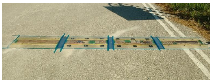
Figure 2. Figure shows the four (4) parts of the “strip” and a typical horizontal installation in the road lane; source [16].
