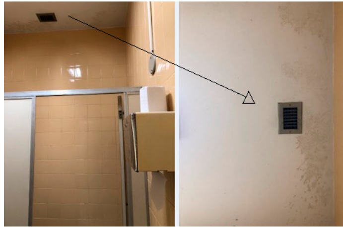
Figure A4. Toilet without window and with an inoperative exhaust fan.
