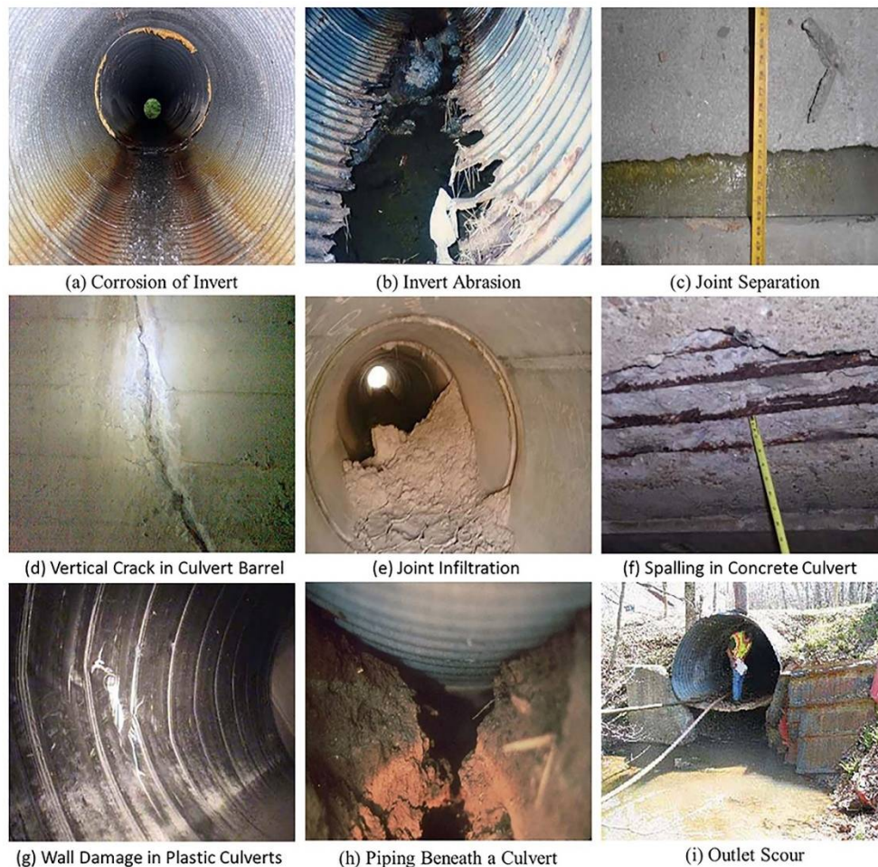
Figure 1. Common defects observed in culverts.
