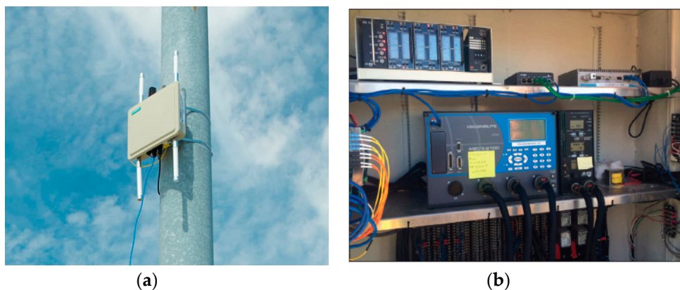
Figure 4. Connected and Automated Vehicle (CAV) elements on the infrastructure: (a) Roadside Unit (RSU) [14]; (b) traffic signal controller [15].
