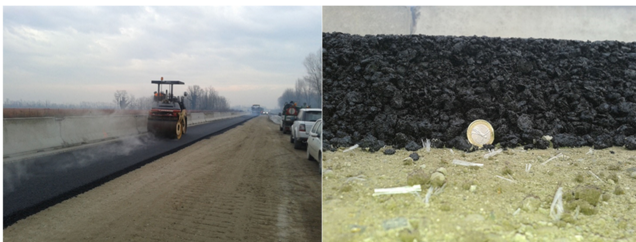
Figure 3. The installation of the base/binder course and its cross-section on polypropylene fiber-reinforced cement-mixed course. The scale coin is EUR 1; 23.25 mm.
