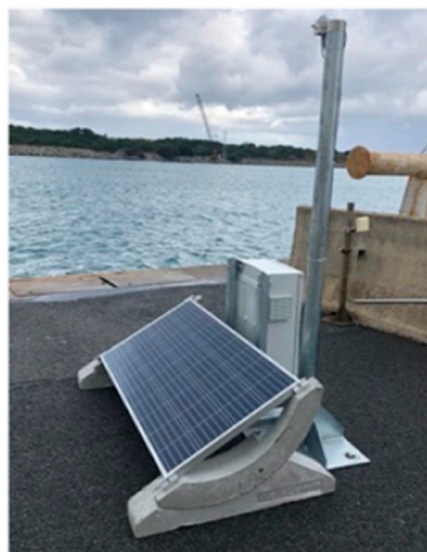
Figure 13. Ground motion and structural monitoring at the port of the Gioia Tauro within the TURNkey project.
