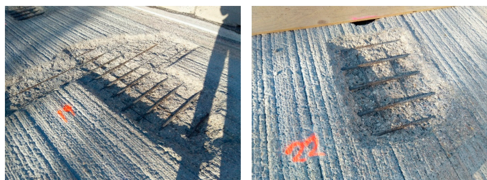
Figure 19. Images showing corroded parts of deck for validating GPR signals.
