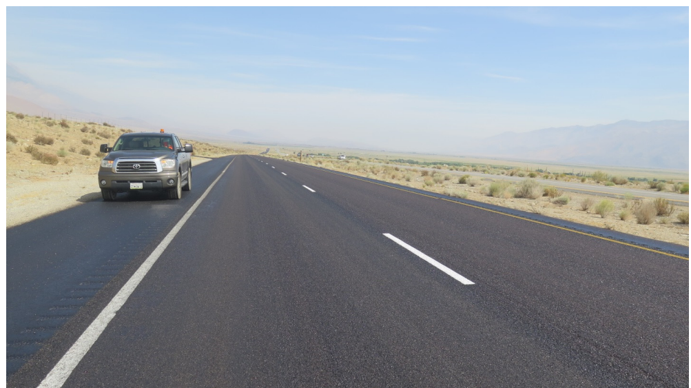
Figure 6. Looking north near south end of project on new double chip seal.
