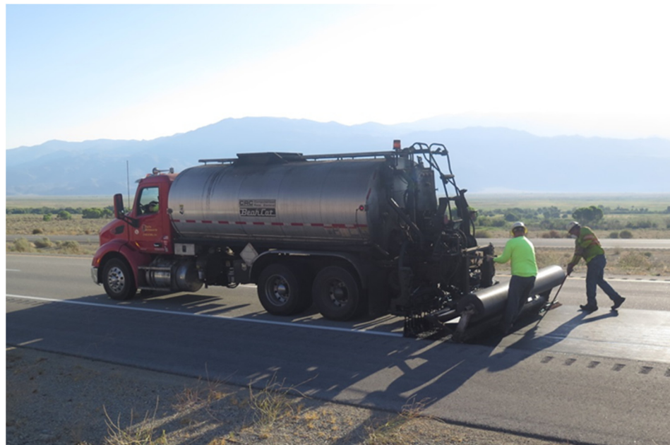
Figure 3. Distributor truck equipped with fabric bracket to apply PG 70-10 binder and paving mat or PRF.
