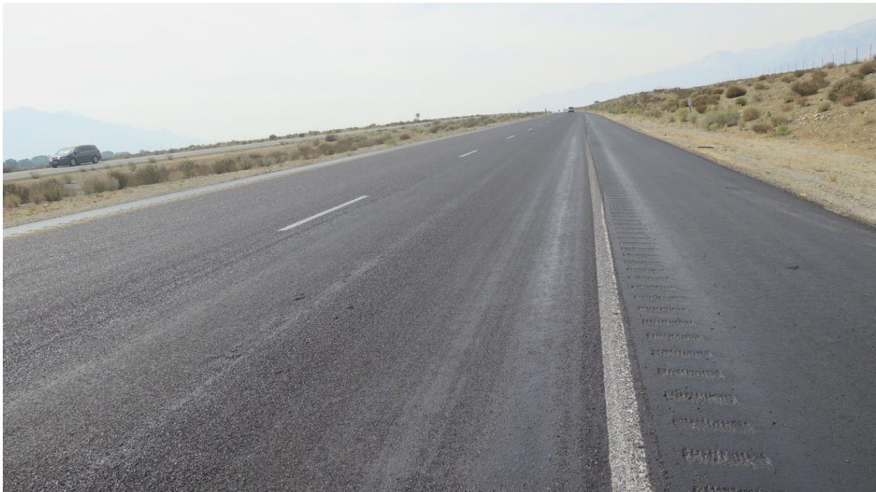
Figure 4. Treatment 2: PME bleeding in right wheel path at PES 4.
