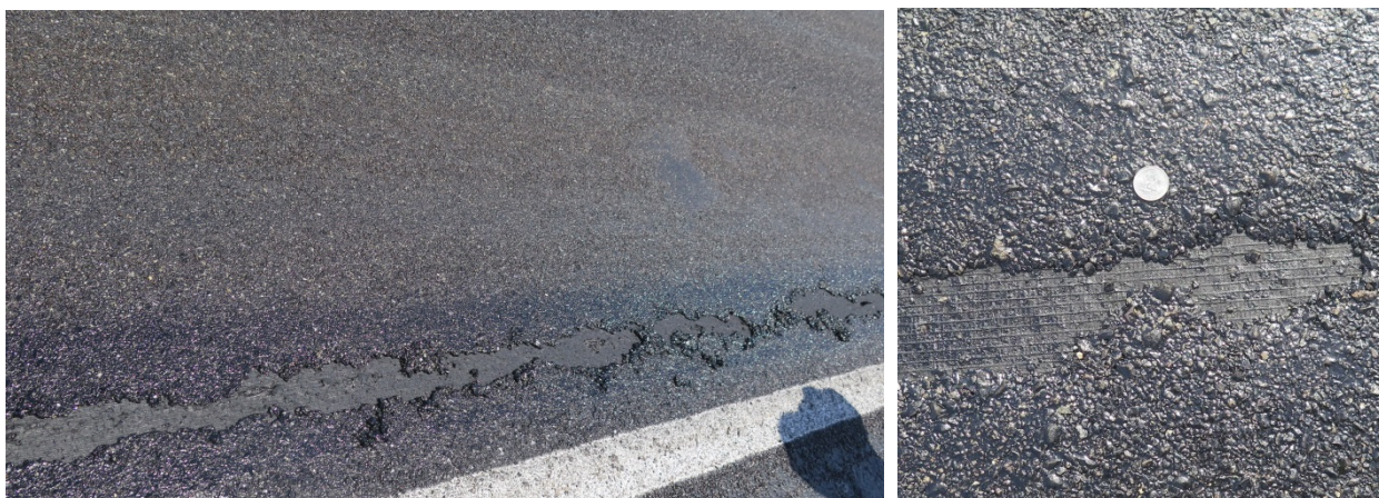
Figure 5. Treatment 3: delamination from GlasPave 50 and bleeding at PES 6.
