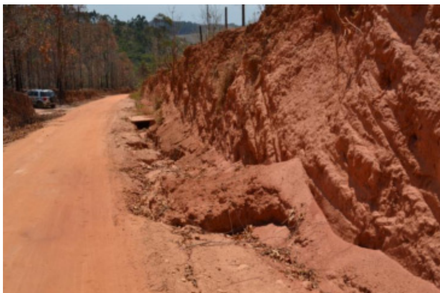
Figure 2. Unpaved road located in the ZMC of MG.
