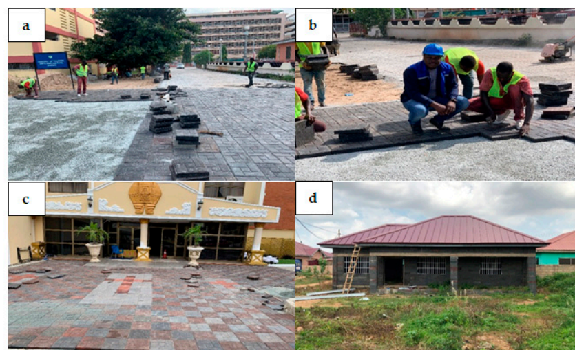
Figure 3. Shredded plastic waste mixed with sand to form pavement blocks. (a) Arranging plastic pavement blocks to lay, (b) plastic pavement blocks being laid, (c) completed laid plastic pavement block, (d) house constructed from plastics. Source: Nelplast Ghana Limited [58].
