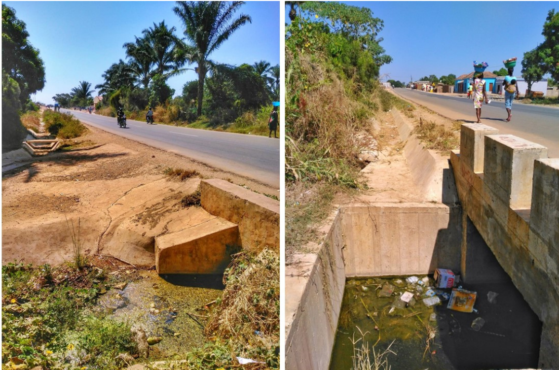
Figure 6. The new road with its drainage water collectors. Observe that in both figures, water is present despite being in the drought season.
