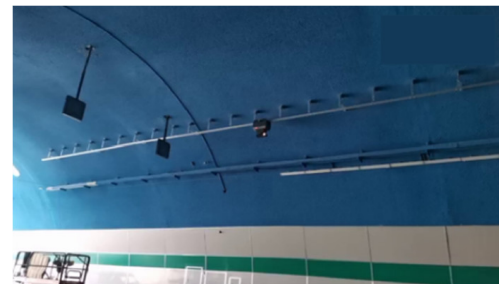
Real tunnel environment (newly constructed tunnel environment, inspection robot track installation height: 6 m)
