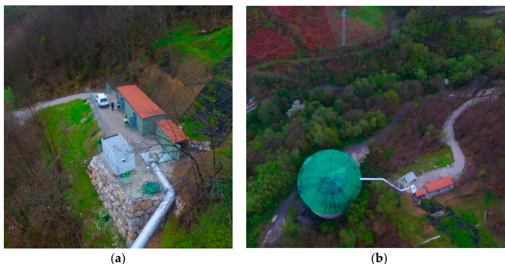
Figure 5. Aerial View: (a) Turbine module and electrical building; (b) The device and the final reservoir.
