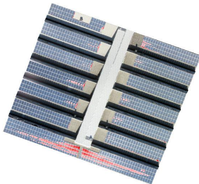
Figure 24. Extracted hotspots and their location within the installation.
