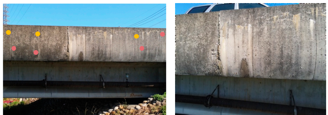
(a) A long-range image covering the control points (pink circles) and check points (yellow circles). (b) A close-up image showing clearer cracks.
