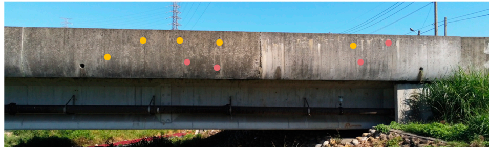
Figure 6. The distribution of control points (pink circles) and check points (yellow circles) on Ai He Bridge.
