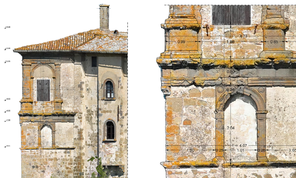
Figure 15. Parts of the elevation on the side of the main facade, redrawn from the integrated digital survey, overlaid on the orthophoto. On the right, a detailed focus of the same elaboration (images by the authors).
