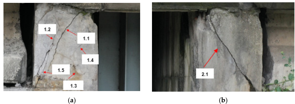
Figure 14. Cracks resulting from shear stress in the head of pier 1. (a) East view, (b) West view.
