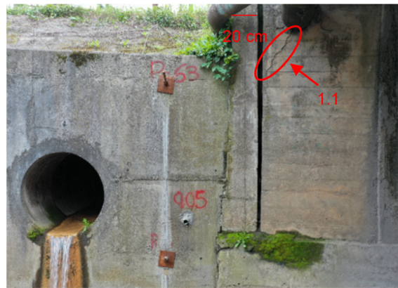
Figure 7. Identification of Crack 1.1 at the small bridge.
