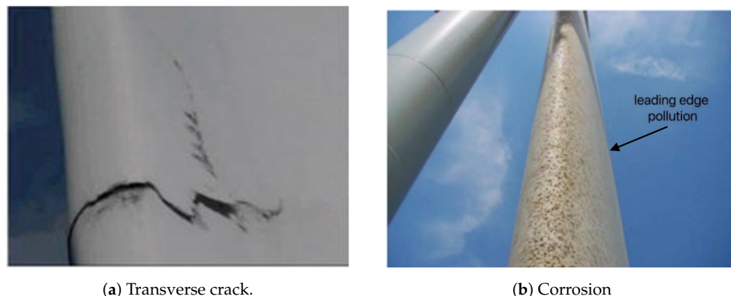
Figure 2. Visual damage examples found on wind turbines (From [42]).
