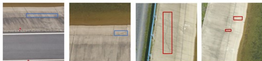
Figure 6. Dam cracks vary widely in shape and size.
